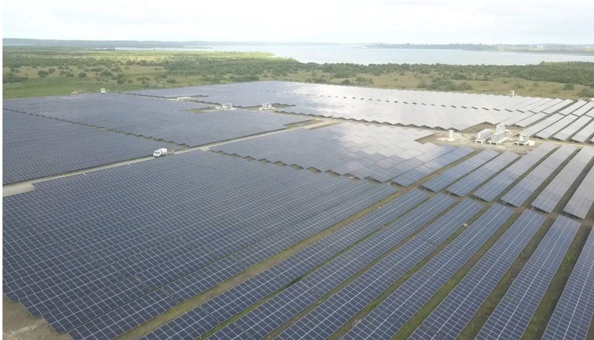
The Corúa 5 solar park in Holguín went online on March 26 (source: Joel Queipo Ruíz/X )
